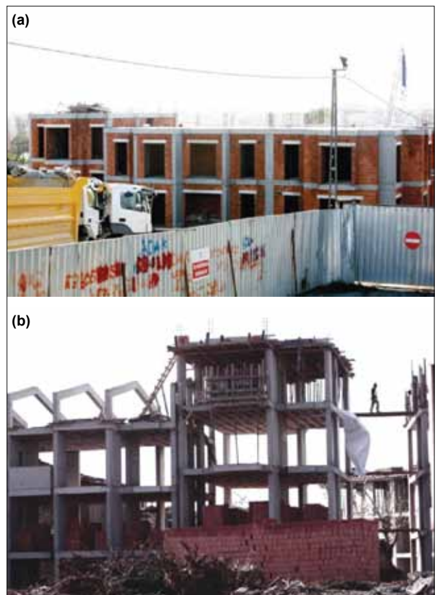
Figure 3. (a, b) Construction of new and quotidian houses in Sulukule. Photograph: Can Berkol, 25.11.2010.
