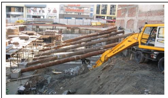
Figure 6. Steel pipe struts were added to give sufficient capacity to the shoring system and to limit the displacements.
