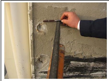
Deformation perpendicular to the excavation (14 cm).
