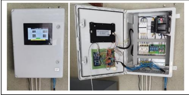
Figure 3. Data acquisition and control panel.
