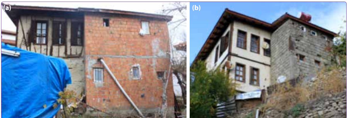
Figure 5. (a, b) Buildings with inconsistently renewed wet places.
