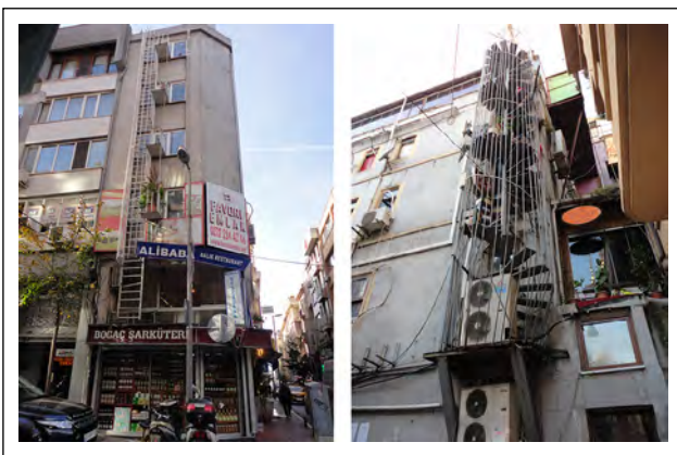
Figure 10. Hazard sources Nos. 4, 13, and 17.
