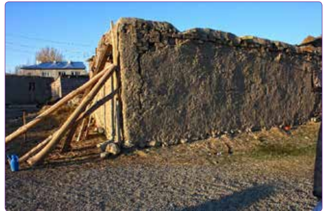
Figure 8. Building which was supported by props after 2011 Van Earthquake (Parsa, A.R. Archive, 2011).
