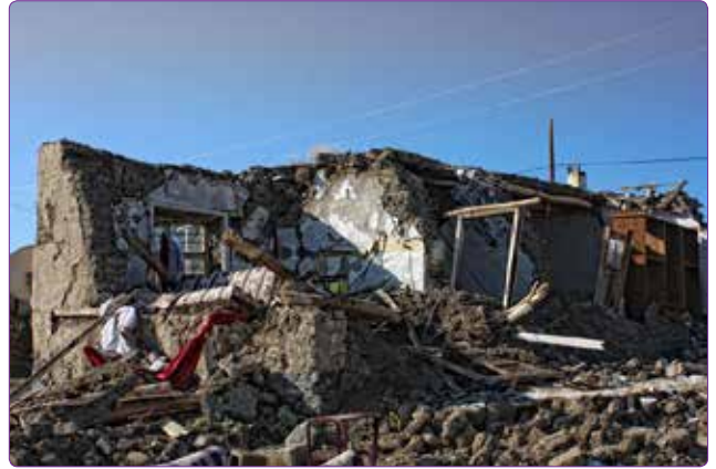
Figure 3. An adobe structure damaged by earthquake as a result of inappropriate material choice (Parsa, A.R. Archive, 2011).
