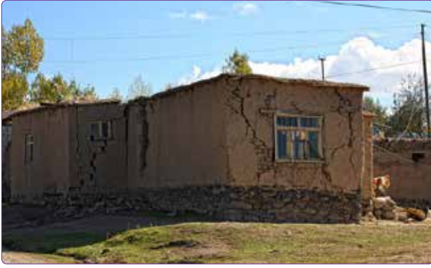
Figure 6. T-Planned structure damaged during the earthquake (Parsa, A.R. Archive, 2011).
