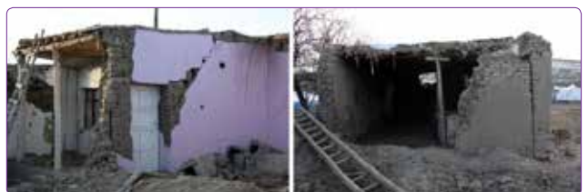
Figure 11. Damaged buildings in the pilot region (Parsa, A.R. Archive, 2011).
