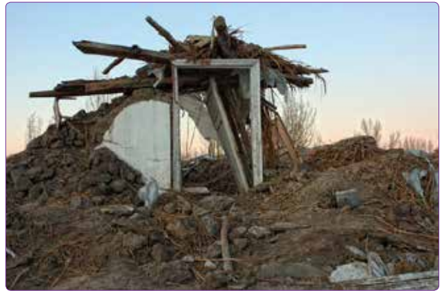
Figure 4. A structure with stone walls, broken down as a result of use of undressed stone and low quality mortar (Parsa, A.R. Archive, 2011).
