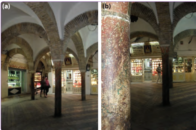
Figure 12. (a) Central area of the covered bazaar, (b) Ropes’ marks in columns (Provided by 1 st author on 20 th of July 2016).
