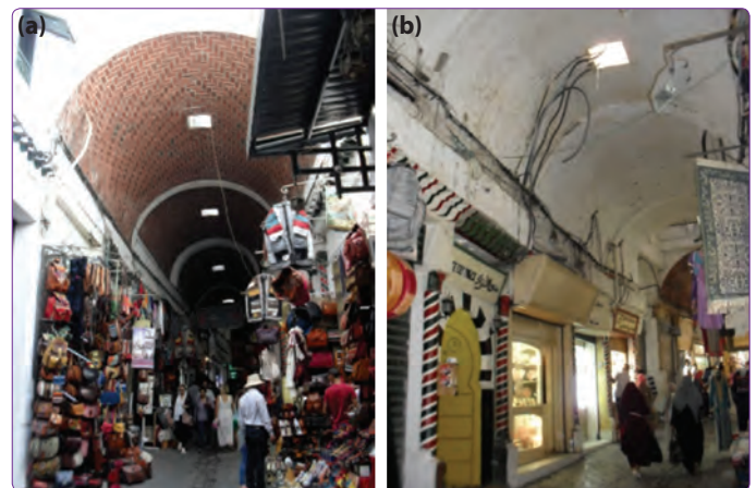
Figure 8. (a) Entrance of "Al-Truk" bazaar, (b) Electricity and air cooling cables in the bazaar's roofs (Provided by 1 st author taken on 20 th of July 2016).
