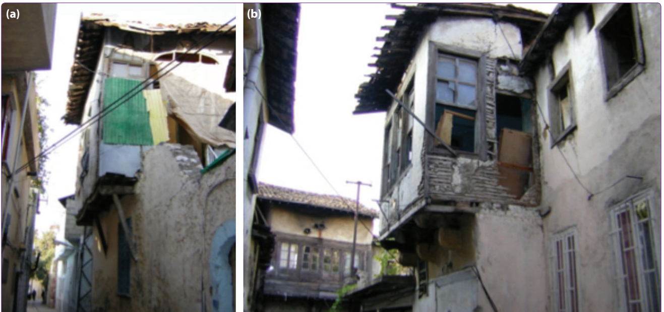
Figure 22. (a) A traditional house in Özdemir Street: An example of a personal attempt to repair an original window (Photograph: Rifaioğlu, M.N., 2005) (b) A deteriorated and vacant traditional house in Sokullu Street (Photograph: Rifaioğlu, M.N., 2005).
