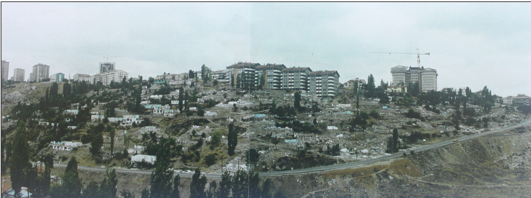
Figure 2. Demolitions of the Squatters in the area reserved for the GEÇAK RP2 (A view from the opposite side of the Valley).
