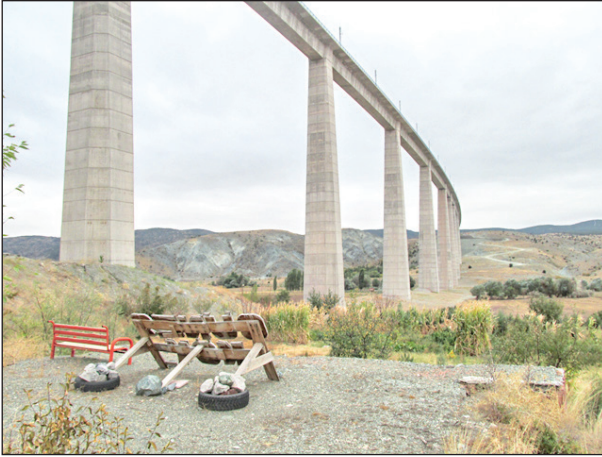
Figure 8. The rail line construction into Güneşköy farmland. Photograph: Valerio Colosio, Esra Demirkol Colosio, 2022.
