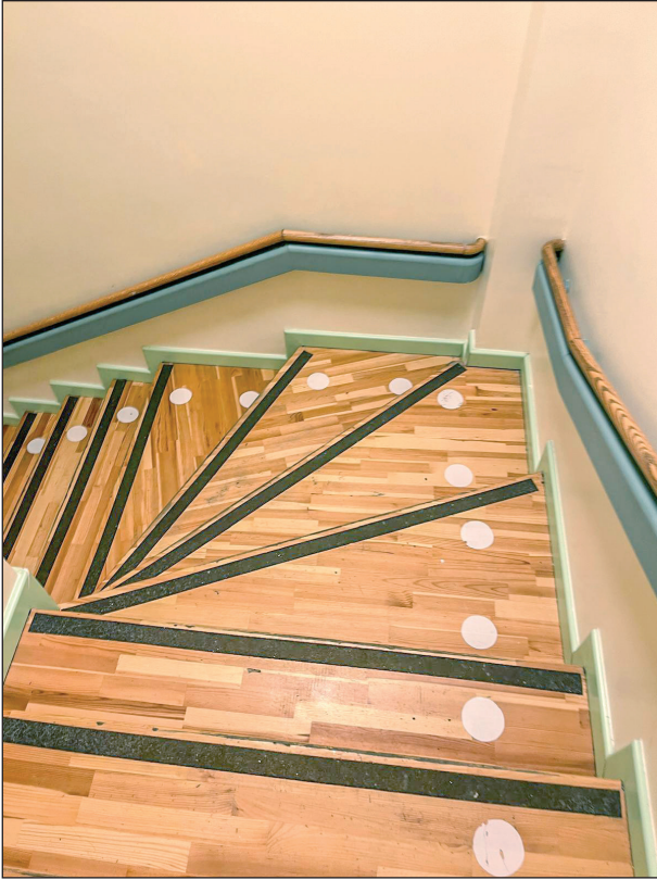
Figure 7. The dining hall staircase at Ayser and İhsan Doğramacı Kindergarten. Photograph: Sera Gülnar.
