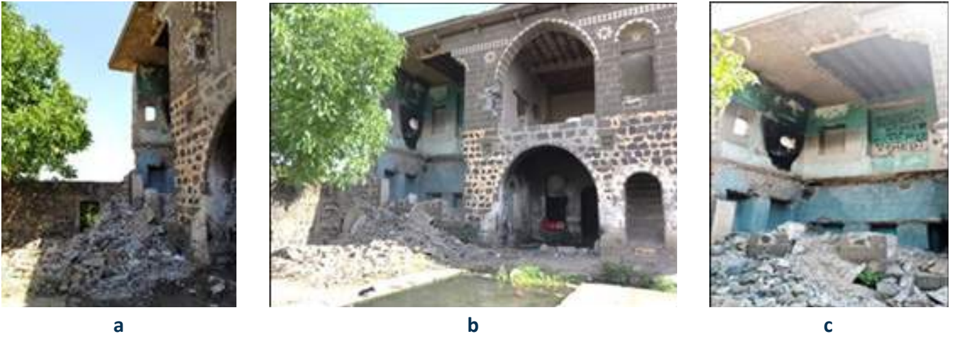
Figure 8. Damages on the northeastern wall of Ferit Köşk (Mansion) (Işık, 2021)
