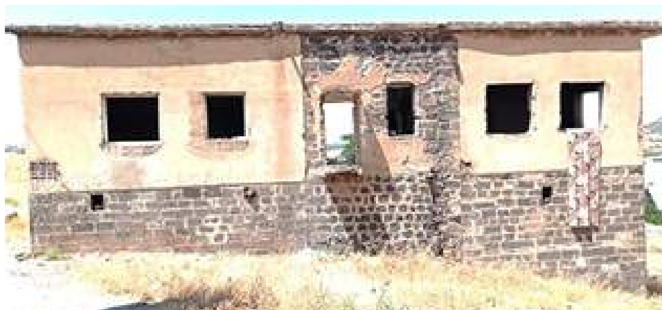
Figure 13. Damages on the southern wall of the Ferit Köşk (Mansion)( Işık, 2021)
