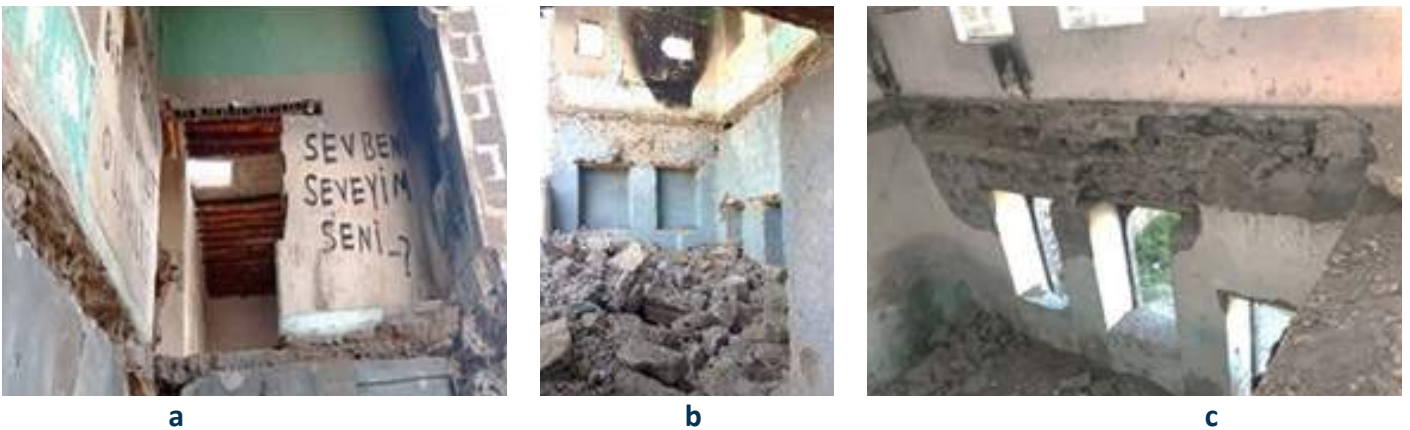
Figure 9. Ferit Köşk (Mansion) floor damages (Işık, 2021)
