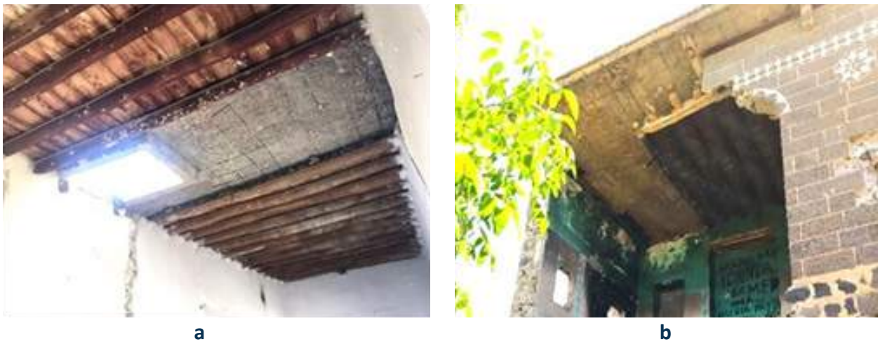
Figure 12. Deflection and material loss damages in wooden beams (Işık, 2021)
