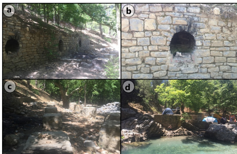
Figure 7. Some neglected structures around the waterfall, landscaping and waste problems.
