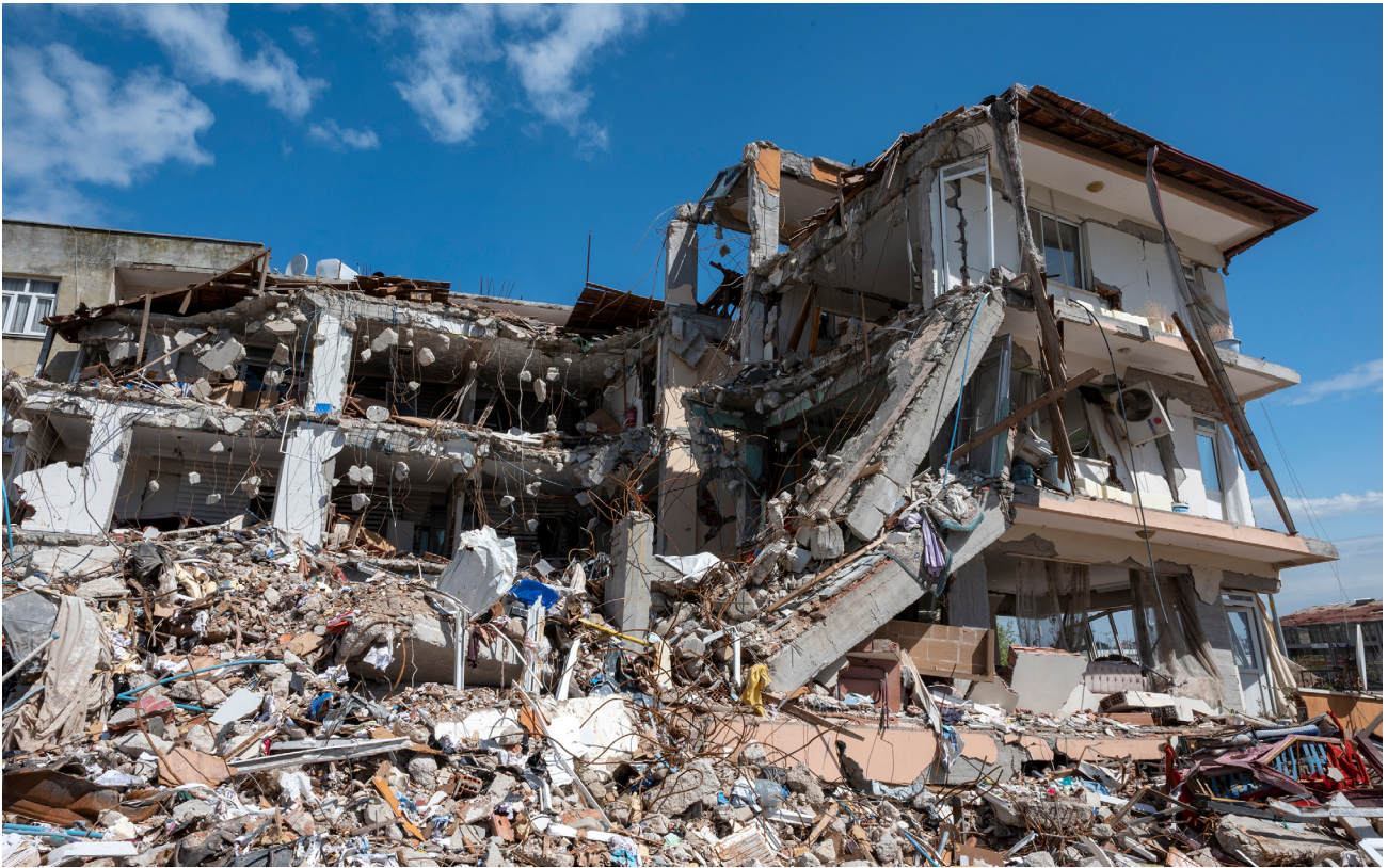
Figure 1. A view from Hatay after the earthquake. (With permission from Dr. Murat Ünal).
