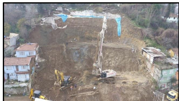
Figure 3. Landslide affected area.
