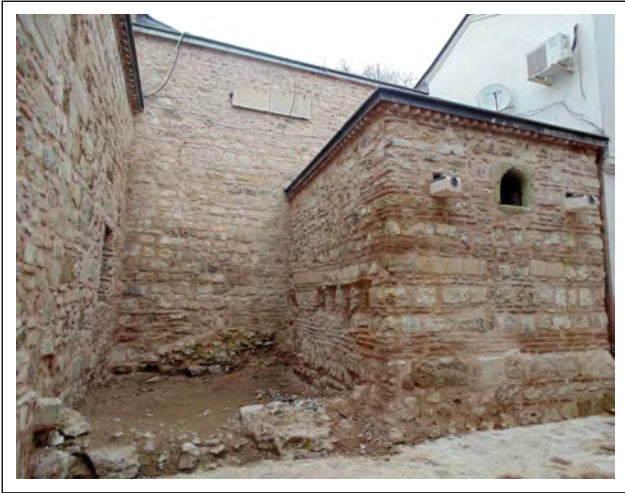
Figure 5. The water tank in kitchen complex, next to the main wall of portico (Uysal Engüdar, 2021).
