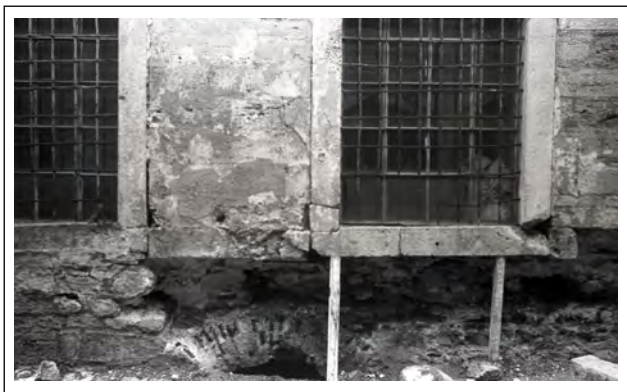
Figure 18. The brick arch on the kitchen’s wall during restoration between 1940 and 1944 (EHAEA, 1940-1944).
