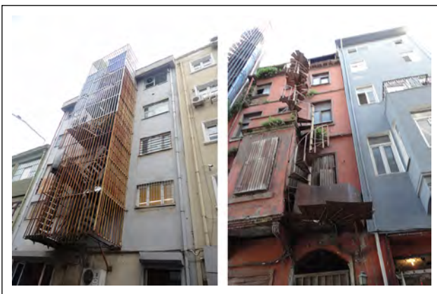
Figure 12. Hazard source No. 15.
