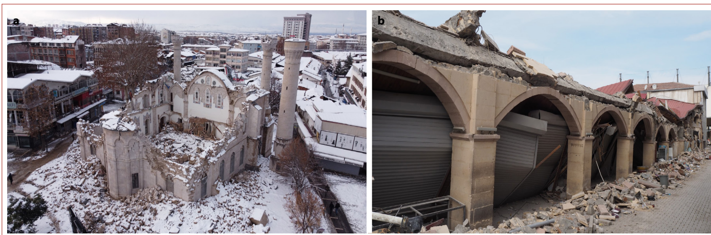
Figure 2. (a, b) City center after the earthquake. (a) Grand Mosque, (b) Grand Bazaar.
